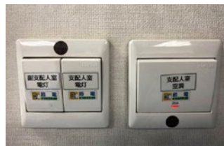
Stickers to prompt energy saving placed on light switches
