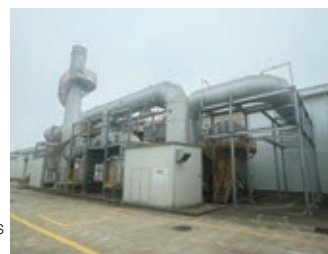
Flue gas treatment equipment at Achilles (Foshan) New Materials Co., Ltd.
