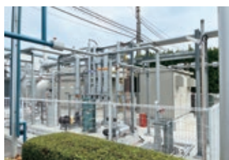
Cogeneration system (Shiga Factory No. 2)
